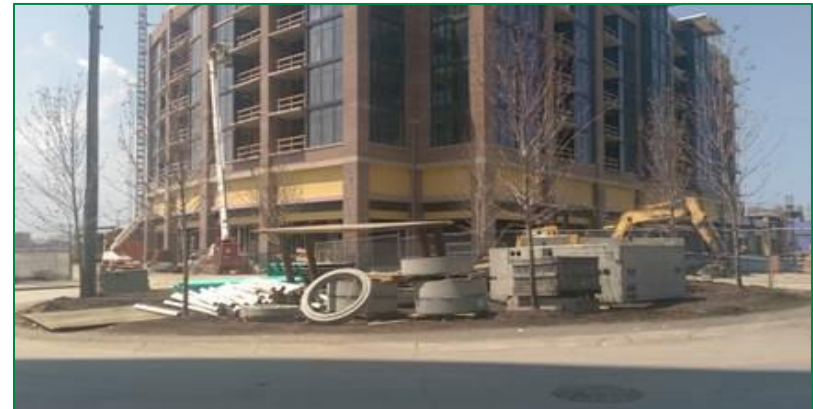
Damage occurs when trees aren't protected during construction. Without significant penalties in place through a tree ordinance, tree mortality in construction will continue and a potential revenue source is not utilized. Image Courtesy of City of Cleveland
